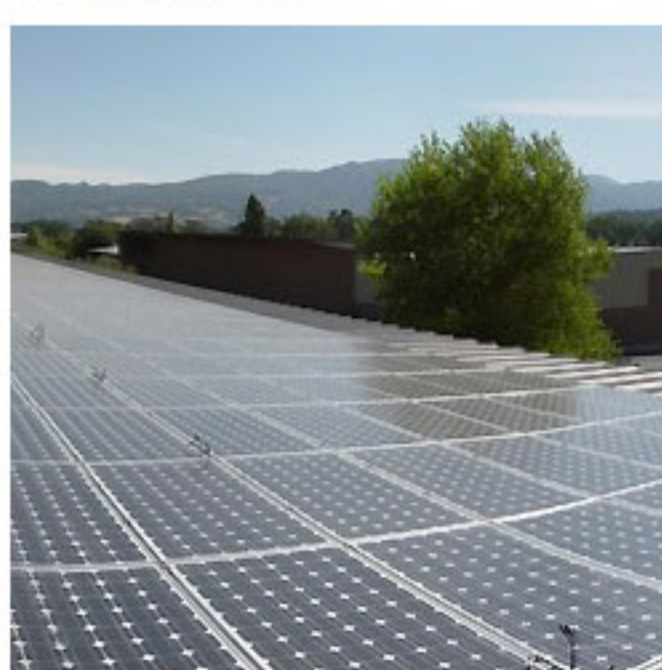
Commercial solar installations relieve stress on the grid.
